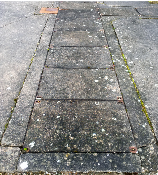
Previously installed concrete infill covers had deteriorated, making covers dangerous to remove, even with specialist personnel and equipment
