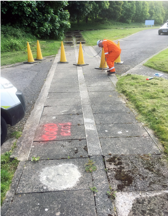
Previously installed heavy concrete covers posed significant health and safety risks
