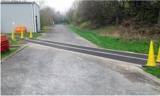
Bespoke Fibrelite GRP composite covers installed at electrical substation in Sheffield
