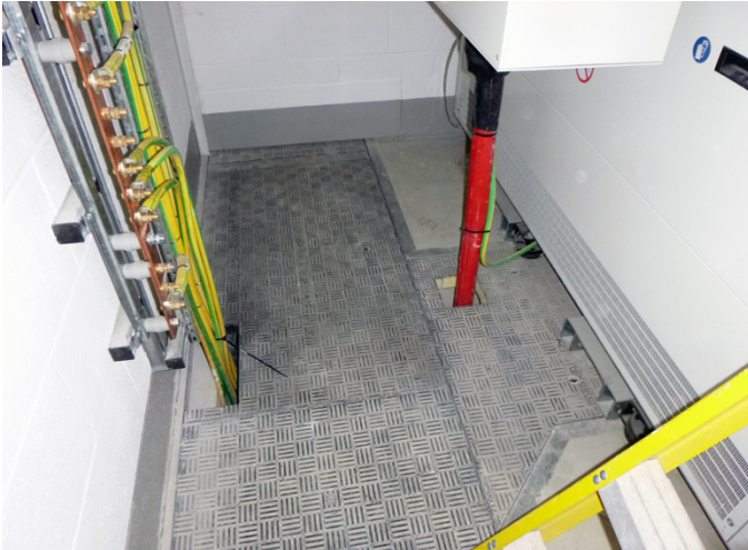
Bespoke Fibrelite GRP composite access covers installed at pharmaceutical facility in County Durham
