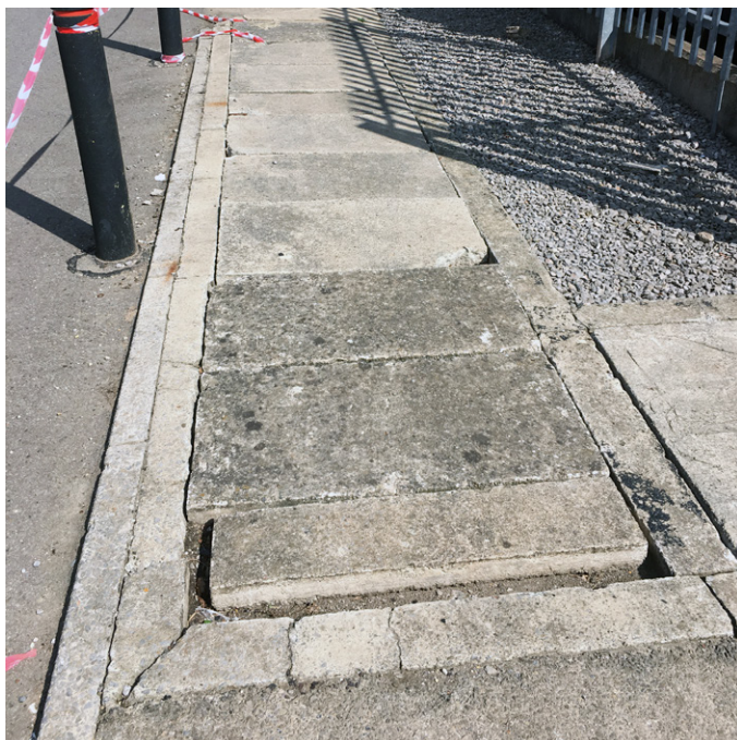
Previously installed failing concrete trench access covers
