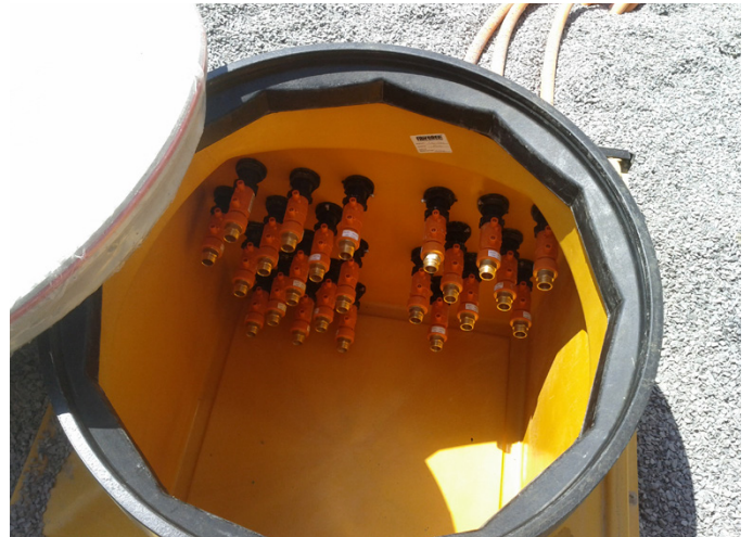
Cable drawpit with 32mm conduit piping
