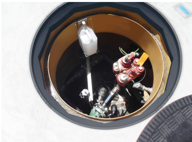
Fiberglass 1.2m (42") turbine sump
