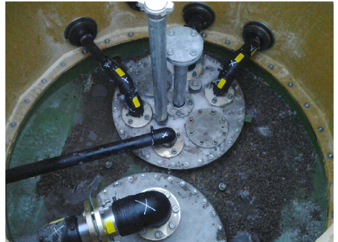
Fibrelite's latest tank sump design installed on CGH Nordic storage tanks
