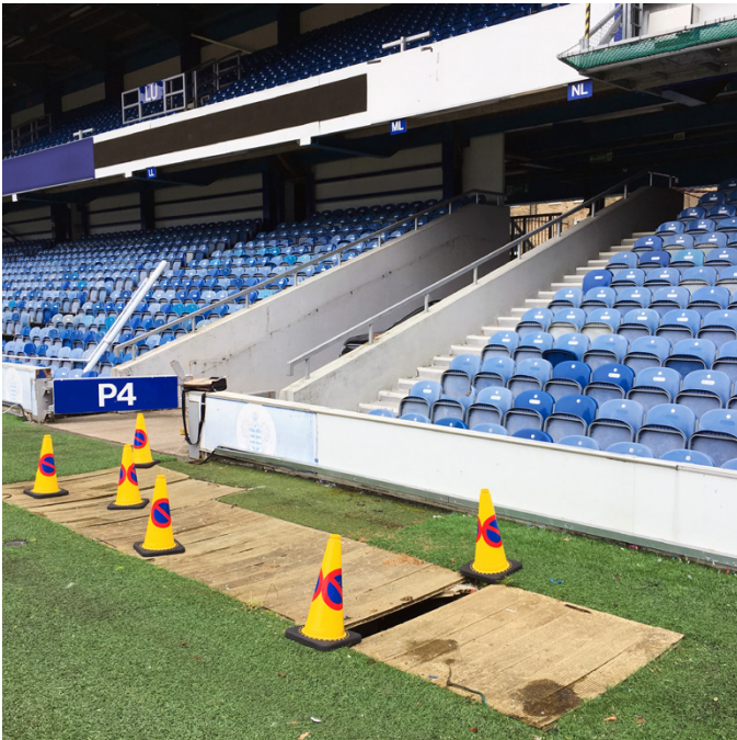
The previously installed makeshift plastic decking had been deemed unsafe for pedestrian use
