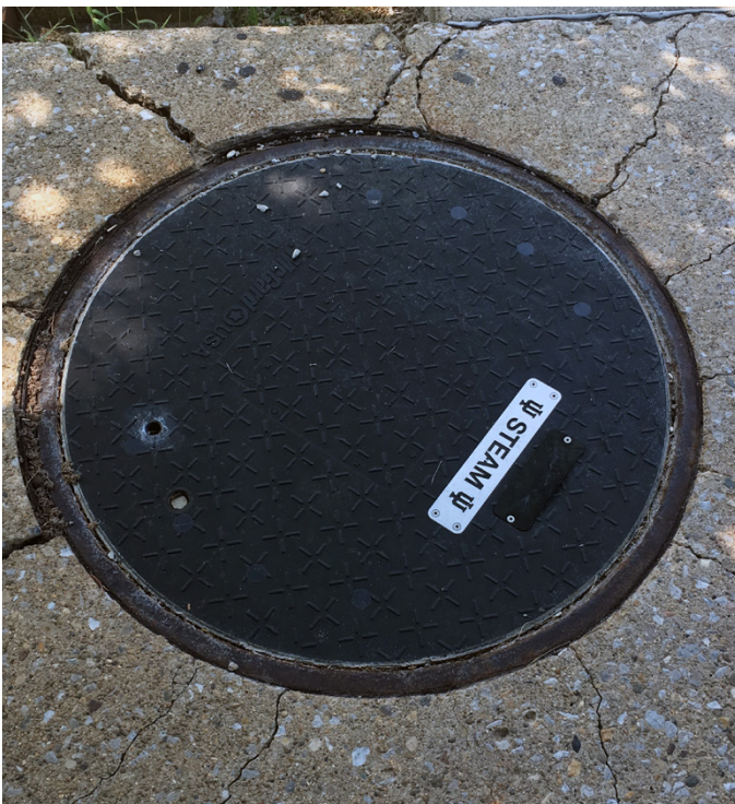
The previously installed covers locking mechanism had failed due to the heat
