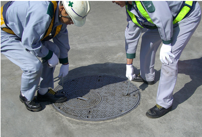
Previously installed heavy metal covers with compromised lifting technique
