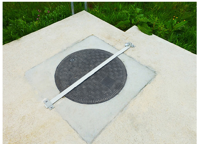
Fibrelite cover with bar installed over for extra security
