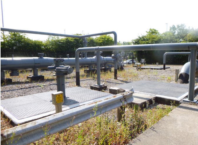
Cadent Gas Valve Pits, North West England
