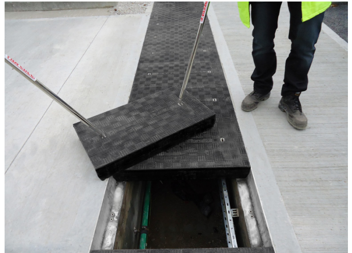
Fibrelite covers are designed to withstand heavy loads and harsh weather conditions for many years (Image of a similar installation used for illustration purposes as actual data centre cannot be shown)
