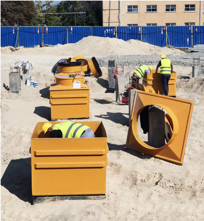
Technical support and installation training was required on site to complete the project within its tight timescale
