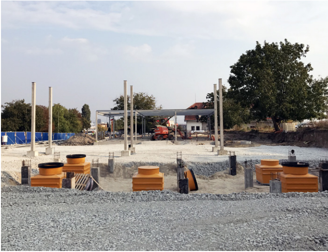
Fibrelite S7-390 GRP tank sumps require minimal maintenance and provide maximum protection (Photo taken prior to KPS pipe installation)
