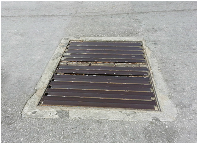
Modular metal covers time consuming and hazardous to remove due to weight, multiple sections and corroded edges
