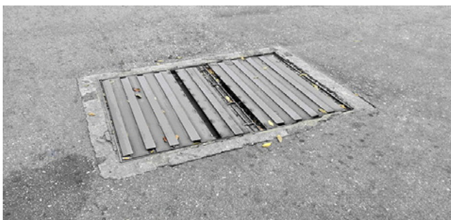
Previously installed steel access pit over water mains valve
