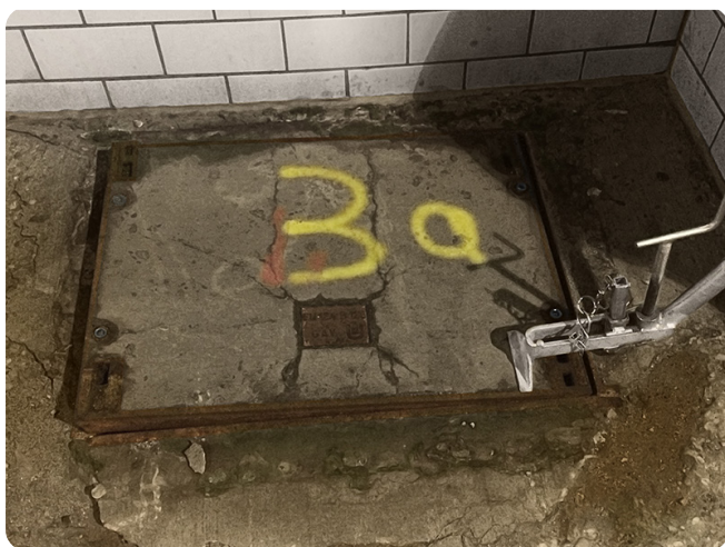
Old unsafe concrete covers
