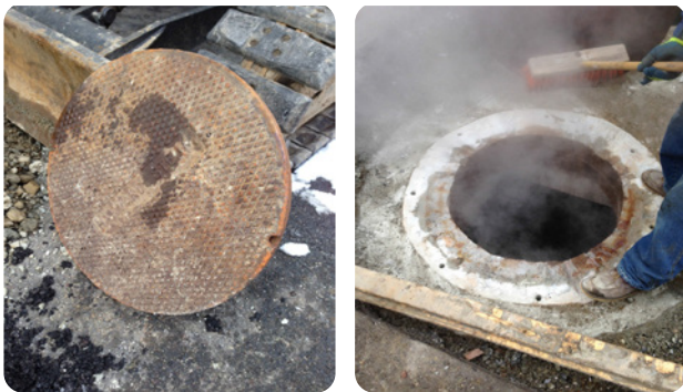
Previously installed large cast iron covers were very heavy and extremely hot when exposed to steam within the manhole
