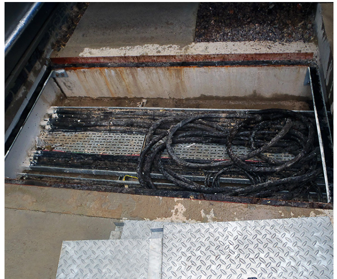
Water ingress due to unsealed covers, causing cable deterioration
