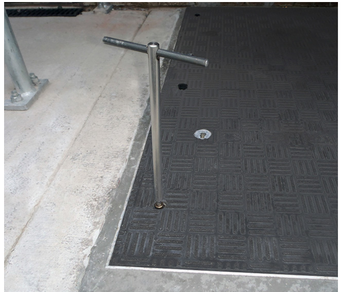
Secured/restrained covers, preventing unauthorised access
