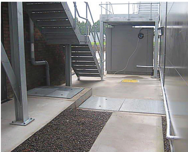
Previously installed steel covers over electrical inspection pit
