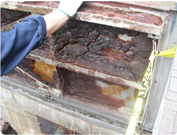
Degraded thermal insulation beneath the old aluminum vault covers
