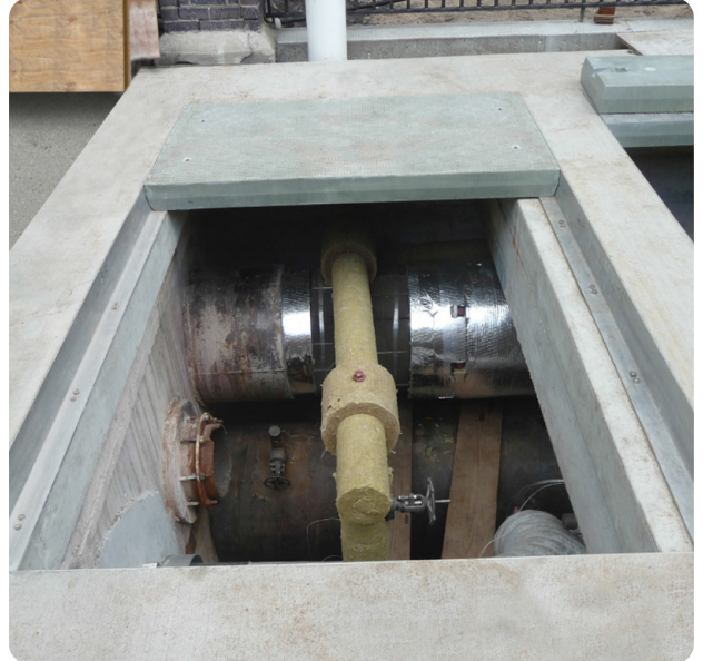
Six Fibrelite FM45 4' 6" (1.6m) wide anti-slip FRP composite trench panels being installed in the sidewalk
