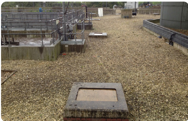
Ease of access: manholes that will soon have a new Fibrelite access cover
