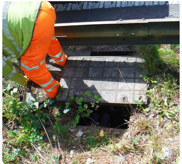
Damaged cast iron and concrete cover
