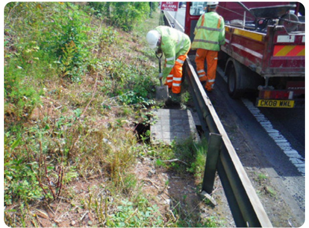
Heavy covers present a hazard for operators
