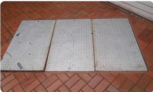
Previously installed odour-emitting galvanised covers
