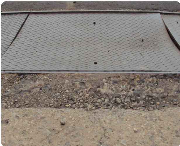
Corroded and deformed: cheap steel covers
