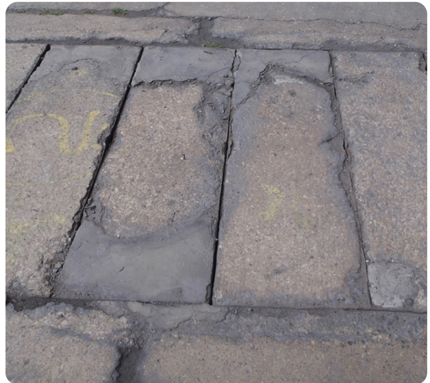
Damaged and difficult to remove: heavy concrete slabs
