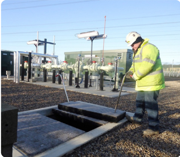
Easy and safe access to underground systems
