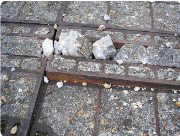
Corroded and damaged cast iron and concrete covers
