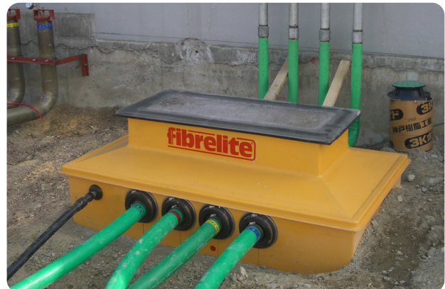
Fibrelite's vapour recovery transition sumps being vacuum tested to ensure a watertight installation
