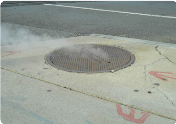
Hot manhole cover on sidewalk poses a threat to pedestrians
